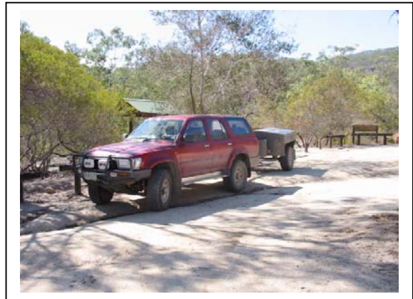
Severe erosion across car park
