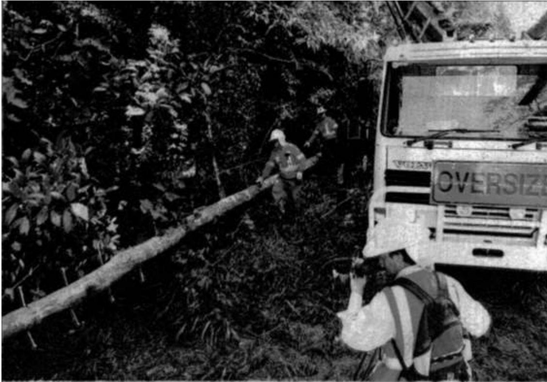
● Ergon workers prepare to erect a pole that will be part of a rope bridge while a cameraman captures it all
